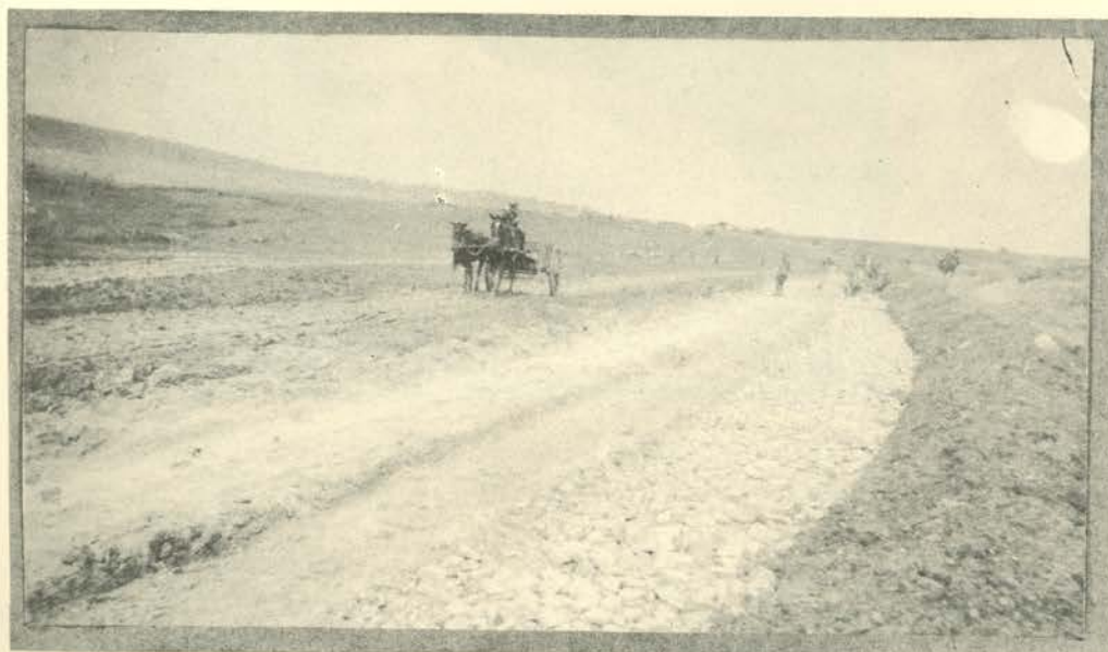
ROAD FROM SAMOGNEUX TO BRABANT REBUILT WITH MATERIAL OF DEMOLISHED HOUSES OF BOTH TOWNS. CONSTANT MAINTENANCE REQUIRED DUE TO HEAVY SHELL FIRE.
