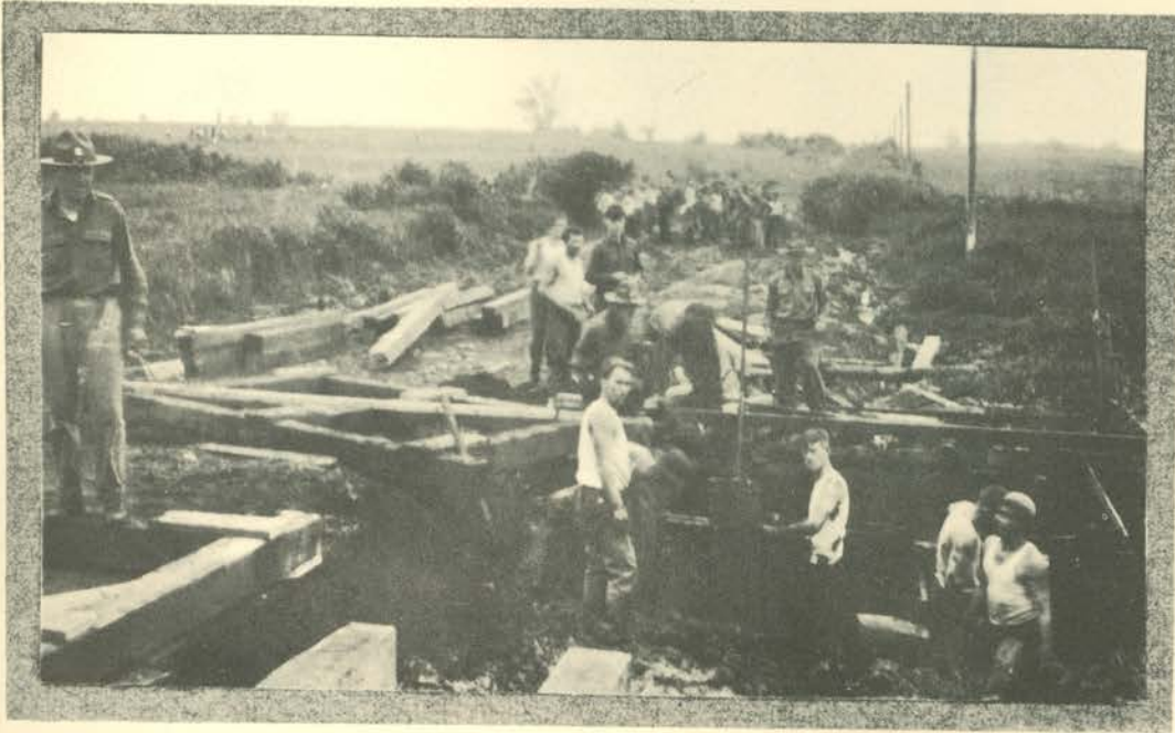
ENGINEER OPERATIONS AT GREGORY FARM. HEAVY BRIDGE CONSTRUCTION. COMBATING SILT AND QUICKSAND.
